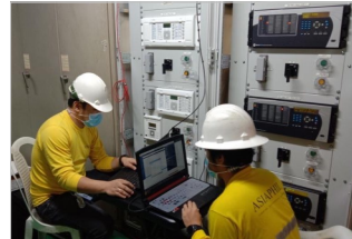
Relay Protection Metering
