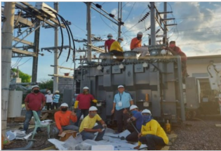
Substation and Grid Connection
