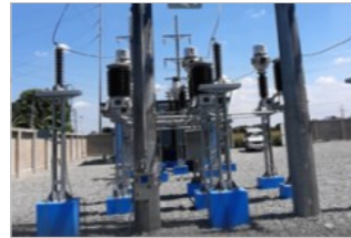
Package 1: 69kV Primary Metering
