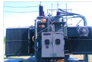
Package 3: Power Transformer (10 & 20 MVA)
